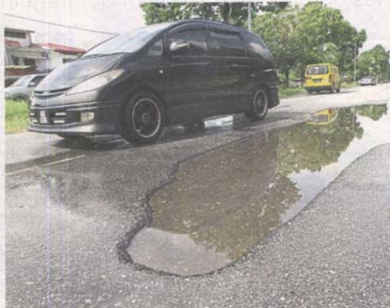
A large pothole along Jalan Gambus in Taman Desawan, Klang. Motorists have to be careful to avoid hitting these potholes.
